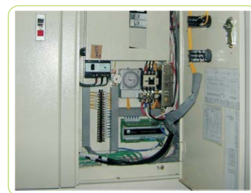
SIO module installed directly in the same panel as the electrical equipment, greatly reducing the cost of labor and work time
