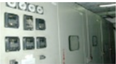
Meter installed at a substation
